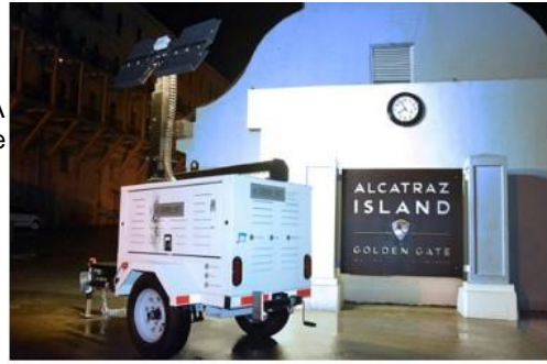
The Zero-Set Lite provides power to critical working lights for an overnight barge exchange operation at Alcatraz Island National Park.
