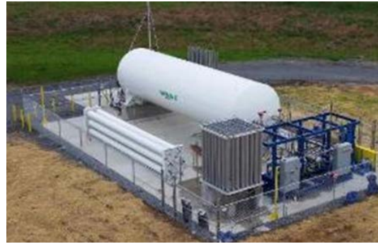
Figure 3 - Plug Power (hydrogen delivery and Storage)
